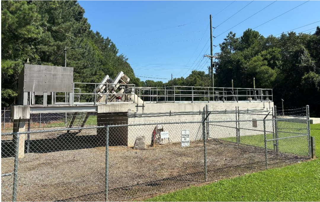
Figure 2 – Cold Water Creek Pump Station
