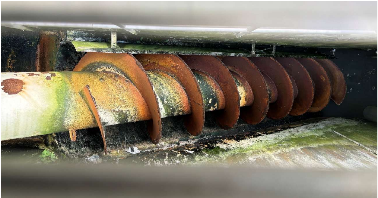
Figure 3 – One of Two Screw Shafts (both in similar condition)
